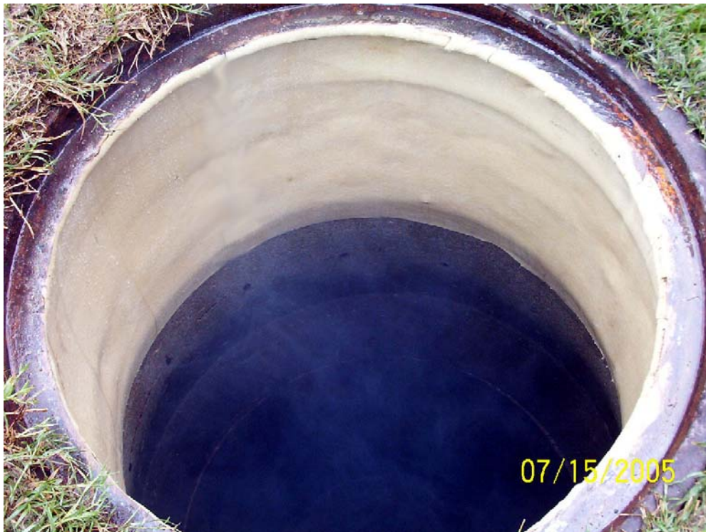
Figure 4. Chimney Liner after First Thaw
