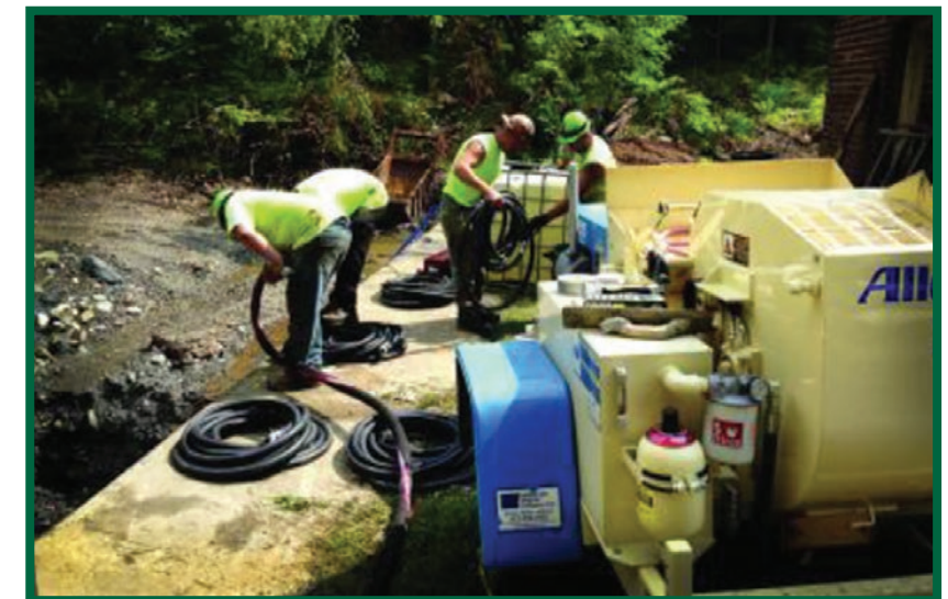
The minimal staging area required made CCCP technology an ideal solution for this project.
